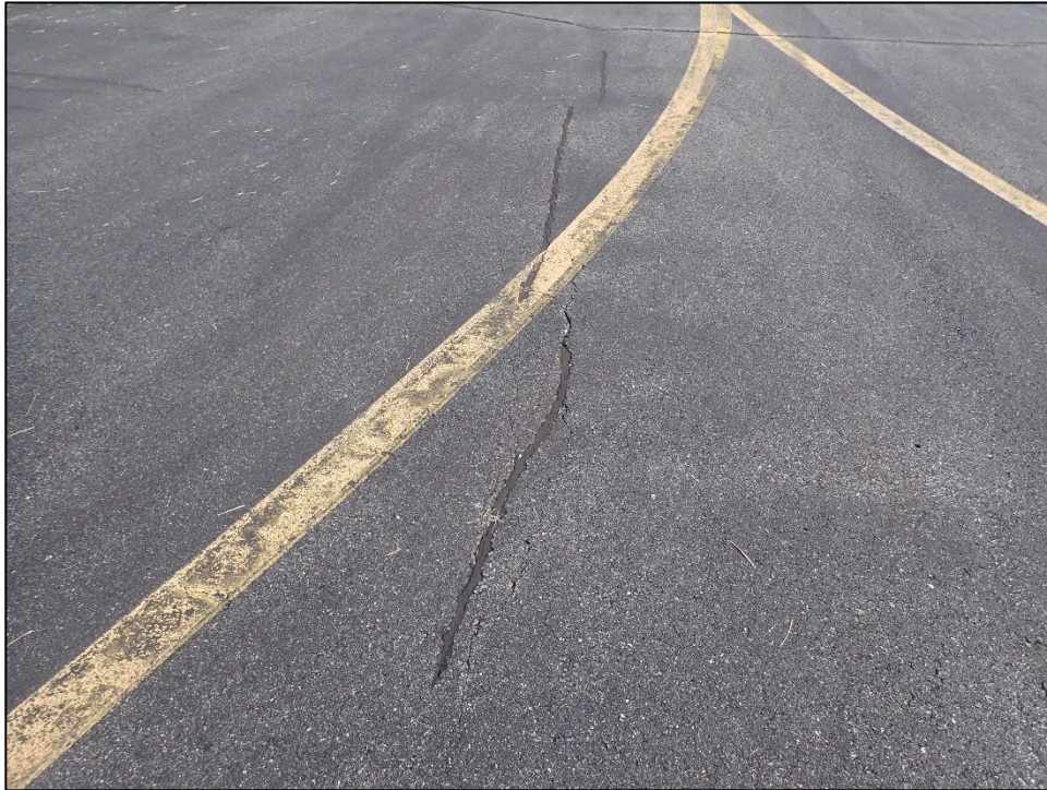
TW-01B-01: L&T Cracking
