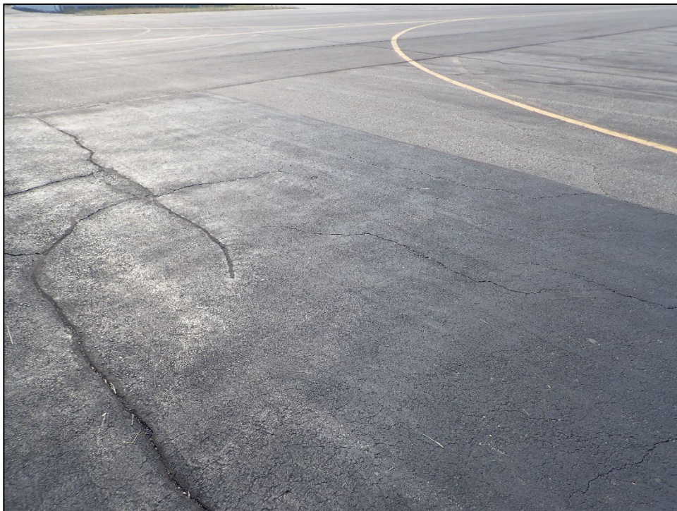
AP-04-03: L&T Cracking
