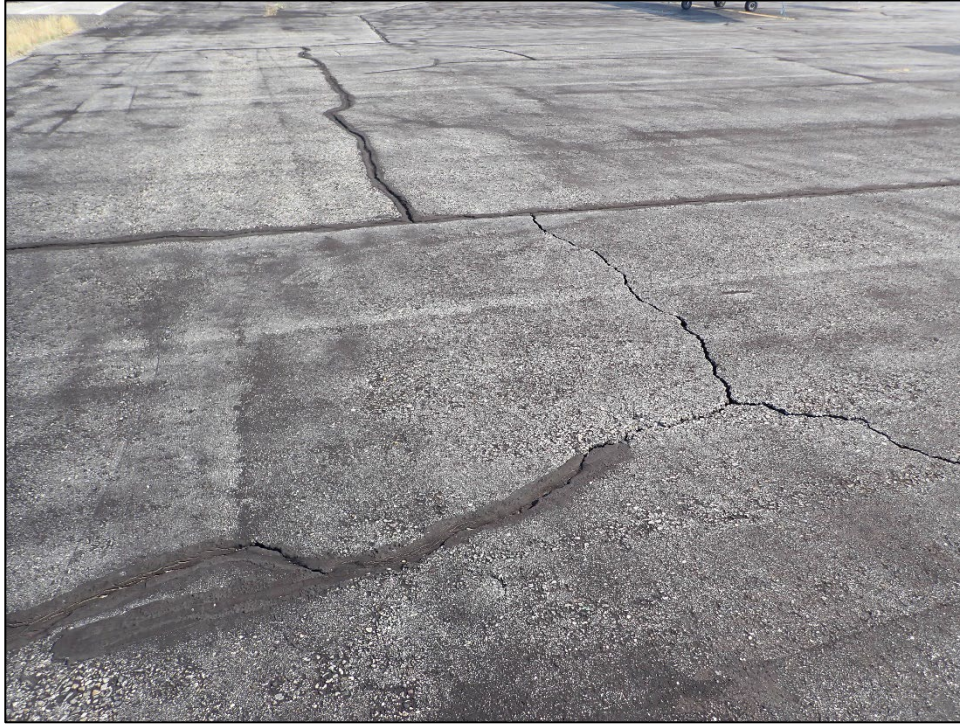
AP-03-09: L&T Cracking
